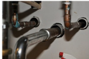
unsealed plumbing (provides entrance)
