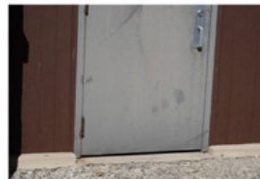
gaps under doors (provides entrance)
