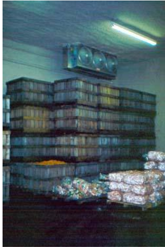
Fig. View of room cooling
