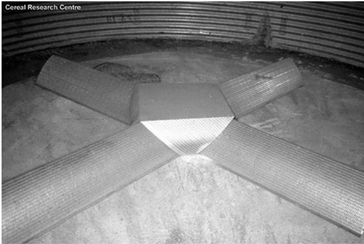
FIGURE 4.50 Aeration ducts in a bin. (From CRC. Agriculture and Agri-Food Canada. Winnipeg: Cereal Research Center.)
