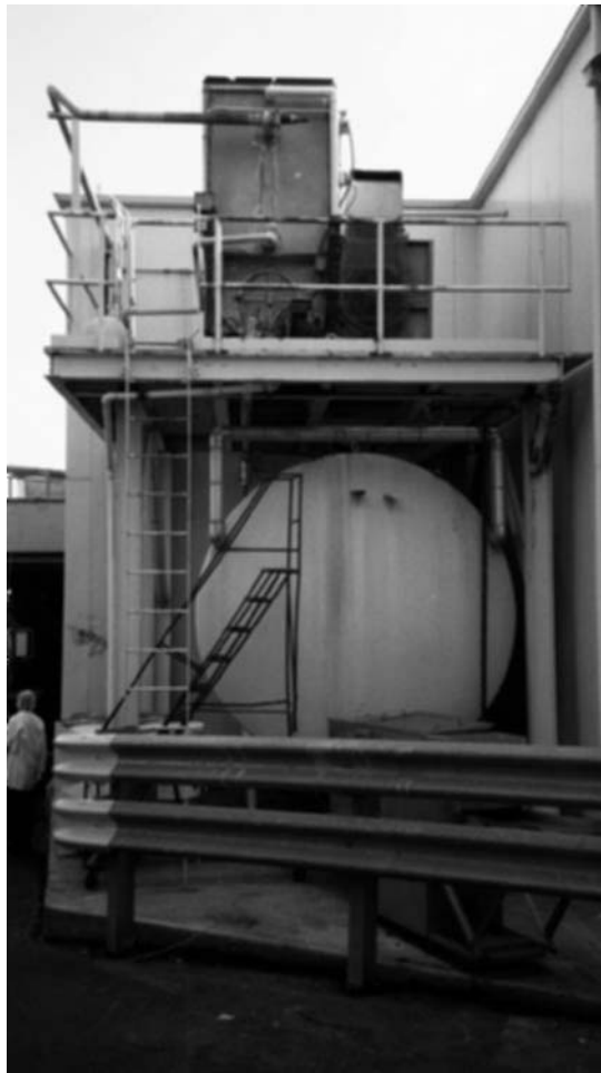
Fig. 10.9 Water prerequisite – cooling water reservoir.
