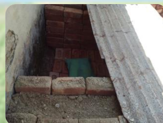
Complete energy cool chamber with shed
