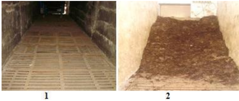
Pasteurization chamber/Tunnel of a Bulk Pasteurization Chamber showing grated panel (1) and compost after phase-I being filled in the chamber for pasteurization process or Phase II (2)
