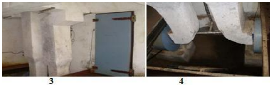
Showing the outer part of a bulk pasteurization chamber with its door closed and air handling unit (3) and the blowers fitted outside the pasteurization chamber
