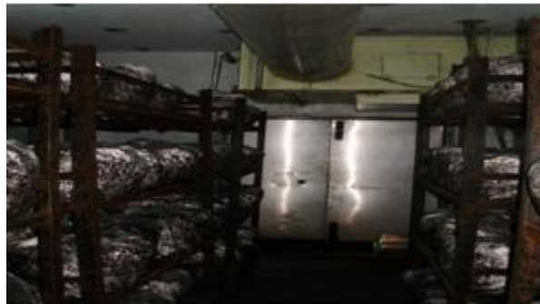
Fig. 11.26 Air handling unit inside the cropping room
