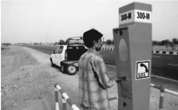
Fig.7.10 : Emergency call box on NH-8
