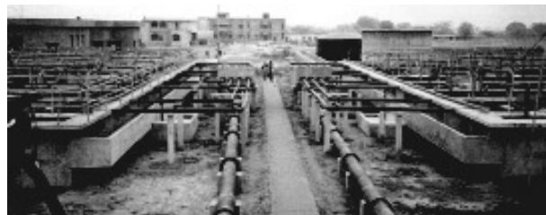
Fig. 6.11: Sewage Treatment plant under Yamuna action pain at Faridabad
