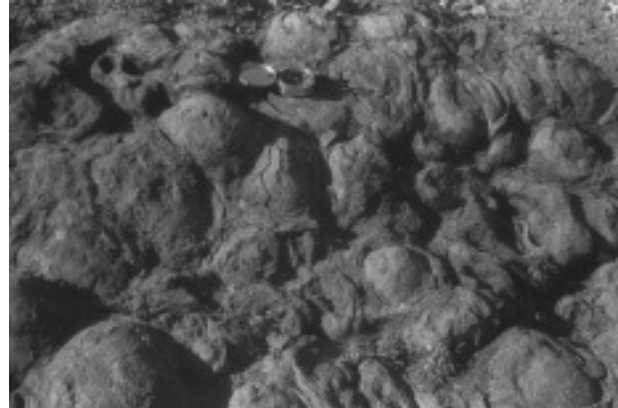
Fig.6.4 : Exfoliation (Flaking) and granular disintegration
