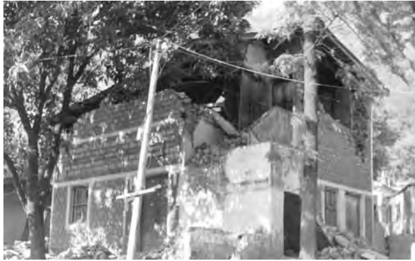
Figure 7.1 : A Damaged Building Due to an Earthquake
