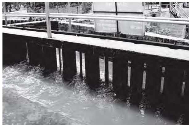
Fig. 18.4 Grit and sand removal tank
